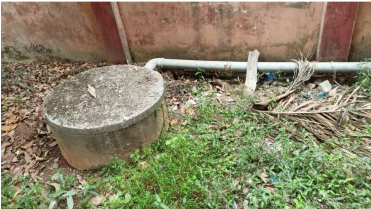
Soak pit for chemical wastes
