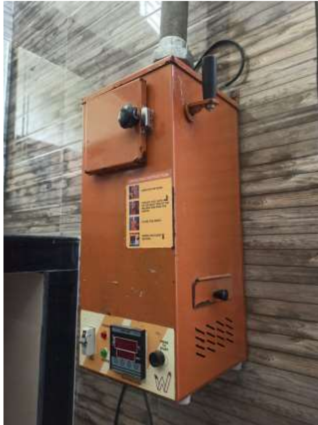
Incinerators for disposal of used sanitary napkins.
