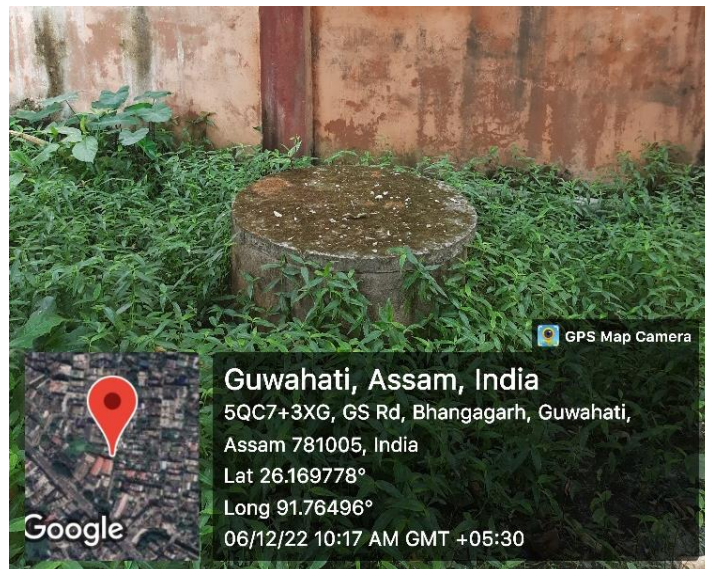
Soak pit for chemical wastes
