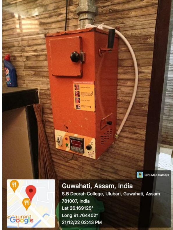
Incinerators for disposal of used sanitary napkins.
